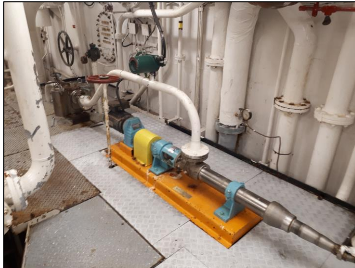
Figure 17. The Moyno pump installed in the engine room (2021, similar for 2022).
