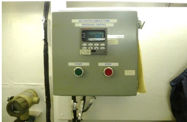
Figure 19. Honeywell controller for the pump, located in the TSG lab.
