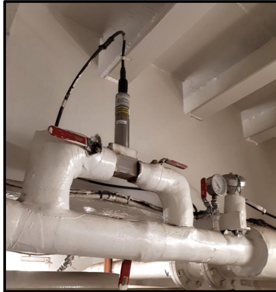
Figure 20. SBE38 temperature sensor in the engine room (2022)
