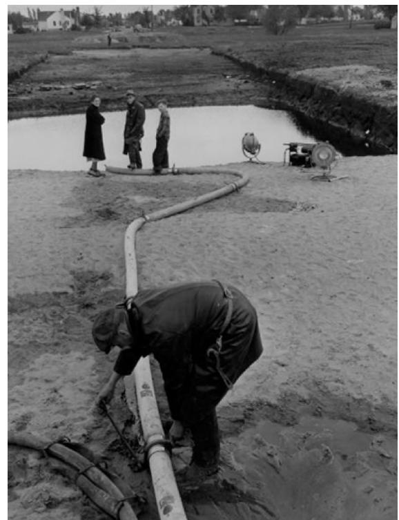
Figure 37: Street Excavation. Pumping out water from a street excavation on 15th Avenue South near 58th Street on May 13, 1941. (Credit: Hennepin County Library, 2021a)
