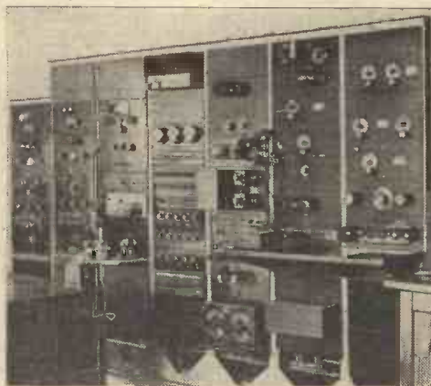
Fig. 3.—Several condenser adjustments are necessary in this intermediate control panel.
