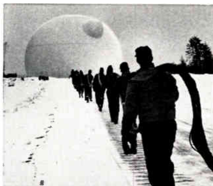
Antenna at the Andover tracking station was erected this winter. Cable is shown being carried during construction.
