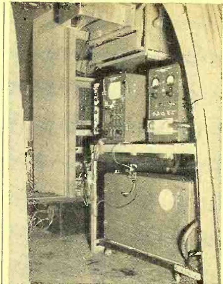
Fig. 4. Rear right interior view shows camera control equipment and synchronizing generator on table; camera low voltage supply is shown beneath table.
