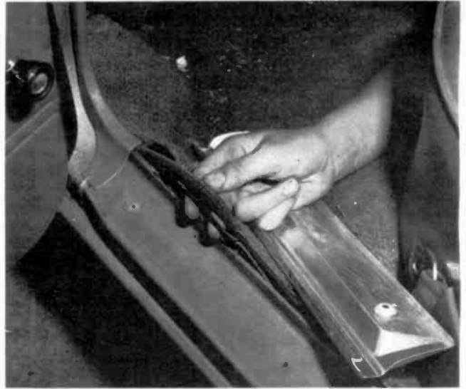
FIG. 6—TRANSMISSION LINE is run from trunk to passenger compartment in wiring-channel under the door saddle.
