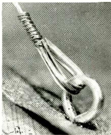
Fig. 8—Screweyes such as this must be screwed in all the way to eye and into solid structural material, not just shingles or decking. Wire here is wrapped only about 7 times; 10 is better. Note ferrule (or thimble) around wire loop, to reinforce it.
