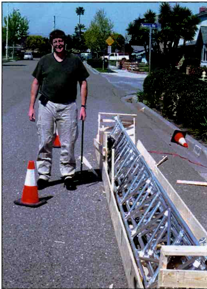
← Don Arnold, WD4FSY, cracks open the crate to get at the tower.
