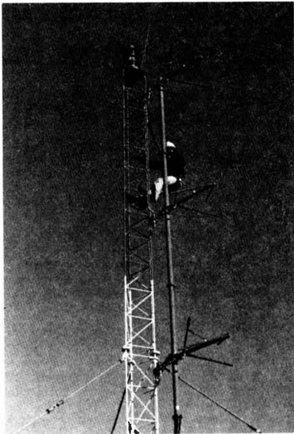
Figure 9. Three bay Cetec model JSCP-3 non-symmetrical FM antenna mounted on the tower leg. The guy cables are insulated fiber glass rods near the tower legs. (Photo courtesy Cetec Antennas)
