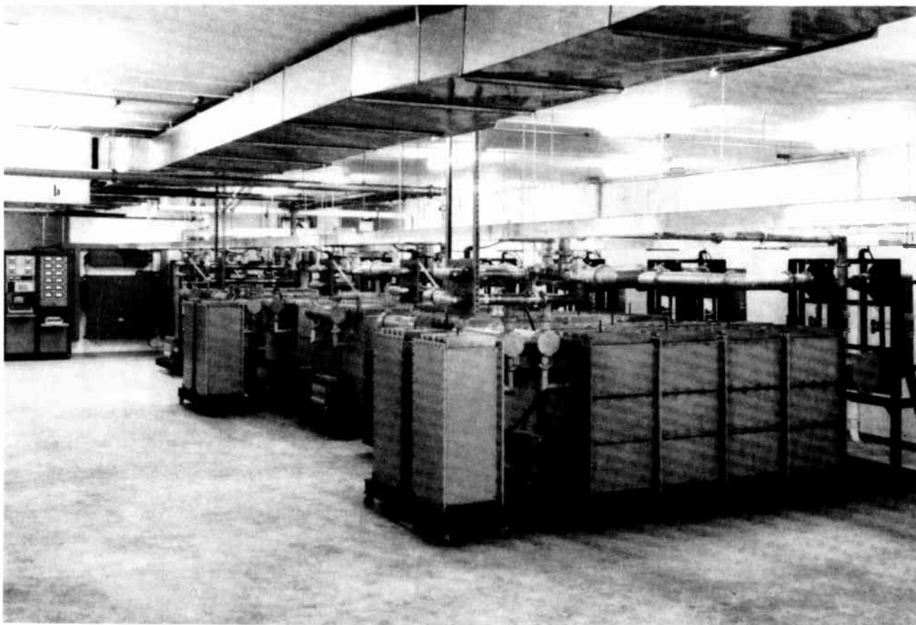
Figure 45. Six-station FM band-pass constant impedance multiplexer at St. Louis. (Courtesy EZ Communications, Inc.)
