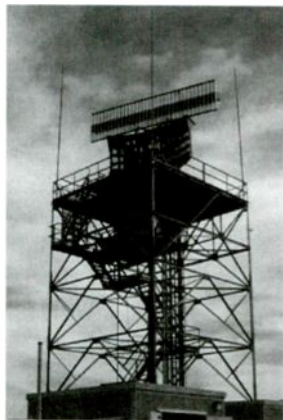
The flat panel Secondary Surveillance Radar (SSR) / ATCRBS antenna can be seen above the primary radar antenna. Both rotate together. (Courtesy FAA)
