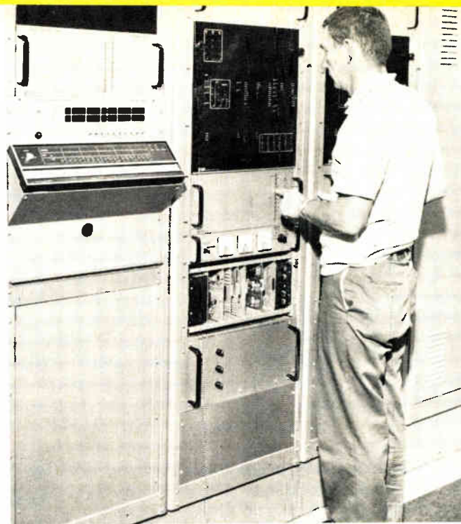
On the rise. U. S. Elevator Co. uses a minicomputer to control its CMC-1200 elevator system.
