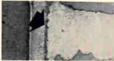
It doesn't take much epoxy to ruin a connection. This discontinuity was caused by smearing of the epoxy during drilling and inadequate cleaning afterward.
