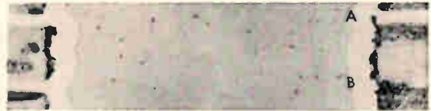
Laminating stresses caused a marginal connection (A) and an open connection (B). However, the flaws do not extend completely around the hole; the comparable connections at the left side of the hole are good.
