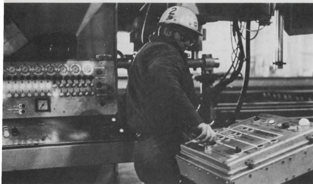
Position holding and welding gantry in the panel shop at Litton in Pascagoula, Miss., assembles stiffeners and T beams into flat panels. The large console (left) controls the gantry and the welding heads. The small one controls the materials passing through the station. Ogden Engineering Corp., Schereville, Ind., built the system.
