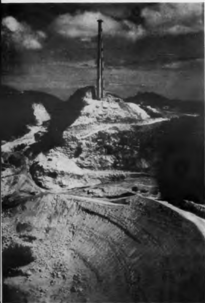
Spherical surface over which a metal mesh will be laid has diameter of 1,000 ft and is several hundred feet deep. Cable-supporting tower rises 250 ft above hill overlooking reflector dish. Tower is one of three to support line feed hanging from a network of cables.
