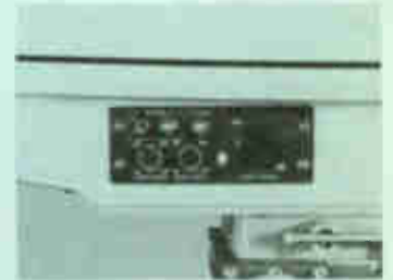
Utility panel provides connections for test equipment and external intercoms, tallies, monitors.
