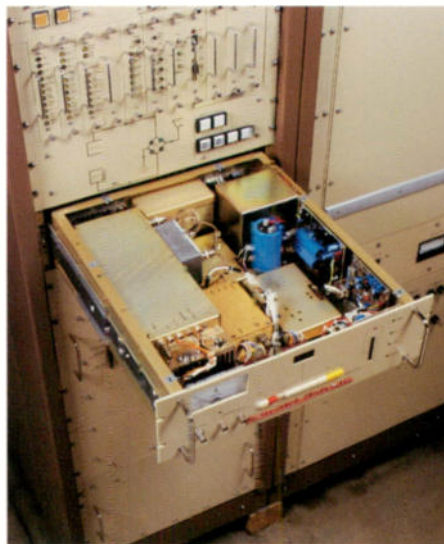
A view of the Exciter drawer in the extended position shows component accessibility.
