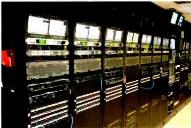
The network went with a traditional master control platform, with a Vizrt graphics engine and Evertz EQX ports for each channel physically mounted in individual racks to ensure channel redundancy.
