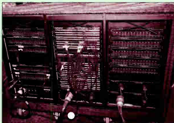
Showconsole audio processing rack. A and B mic inputs for up to 80 channels are input via standard multicore connectors. 80 C inputs are on XLR connectors, and the 80 line inputs appear at the TT patchbay.
