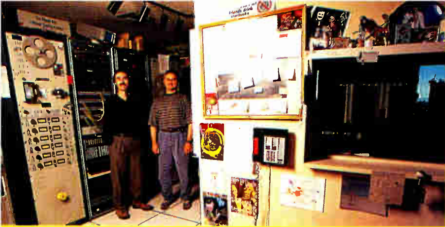
Chief engineer Jim Austin, left, and systems engineer Vince Casper in Transfer B; the Sonic network loading station is pictured through the window at right
