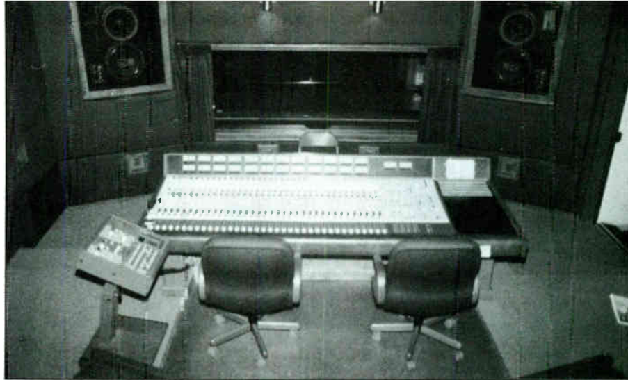
Audiovisions' Control Room A, Louisville, Kentucky
