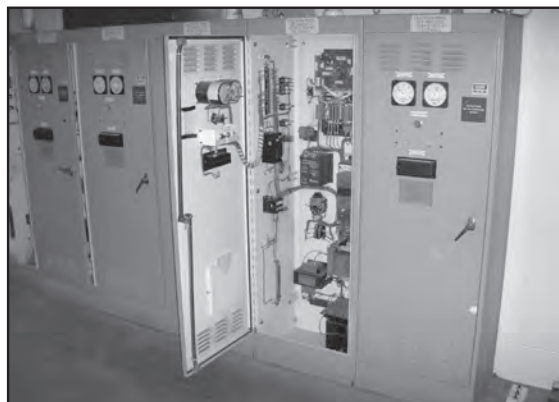
A typical '80s analog exciter control panel crowded with obsolete components
