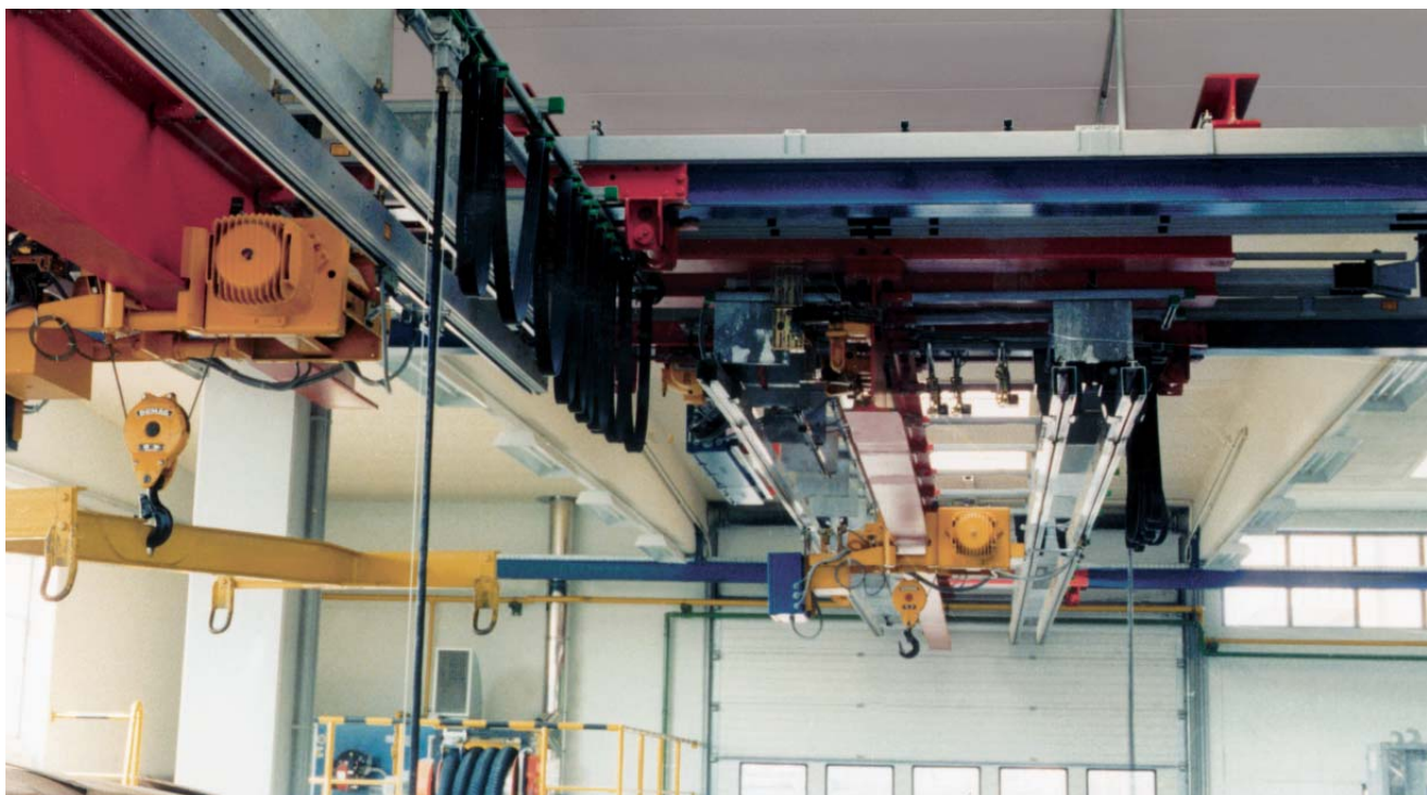
Aluminium enclosed conductor system on crane bridge.
