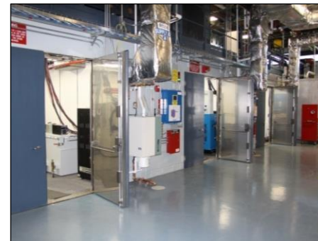
Internal Cell/Module Test Rooms
