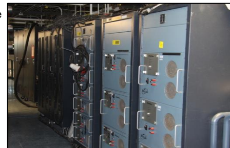
Cell, Module & Battery Cycling Equipment
