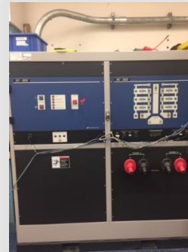
Power Cycling Station
