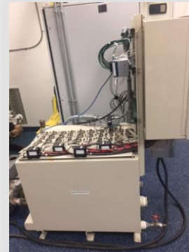
250kW Resistive Load Bank
