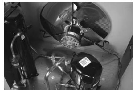
Typical Outdoor Unit with throwaway liquid-line filter and sight glass
