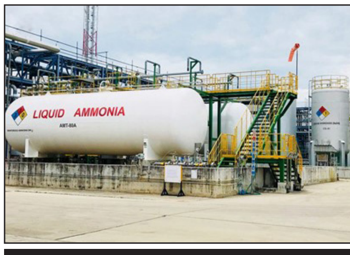
FIGURE 10 Example of Liquid Ammonia Storage [Simon, Taylor, 2021]
