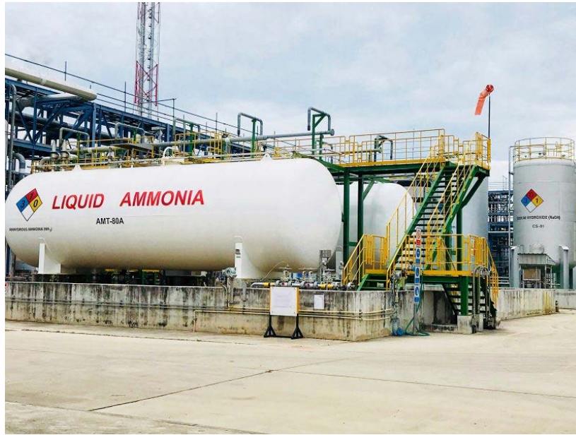
Figure 6.14 Example of Liquid Ammonia Storage [Simon, Taylor, 2021]
