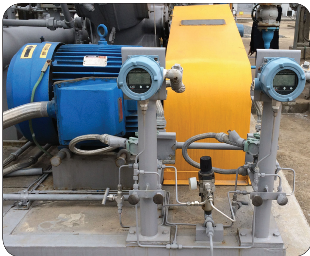
Pump Emergency Shutdown
