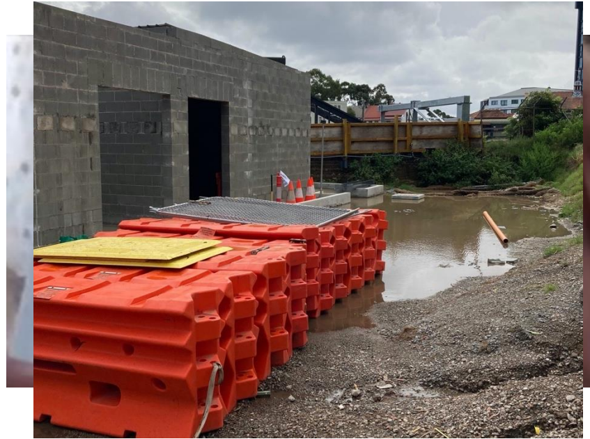
Photo 5 – Water accumulated from continuous rain and ERSED controls in place near SSER Building works on Marian Street compound.
