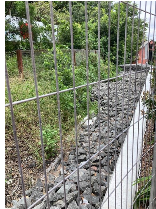
Photo 14 – Vegetation growing around heritage retaining wall in Little Eveleigh Street car park.
