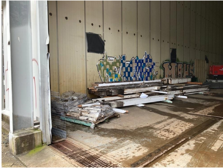
Photo 15 – Storage of timber removed from the 125-127 Little Eveleigh Street, kept for reuse.
