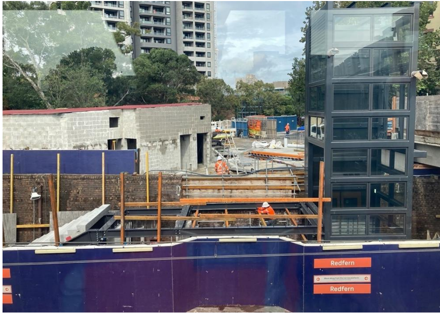
Photo 8 – View of SSER building construction, lift riser installed and stairs works in progress
