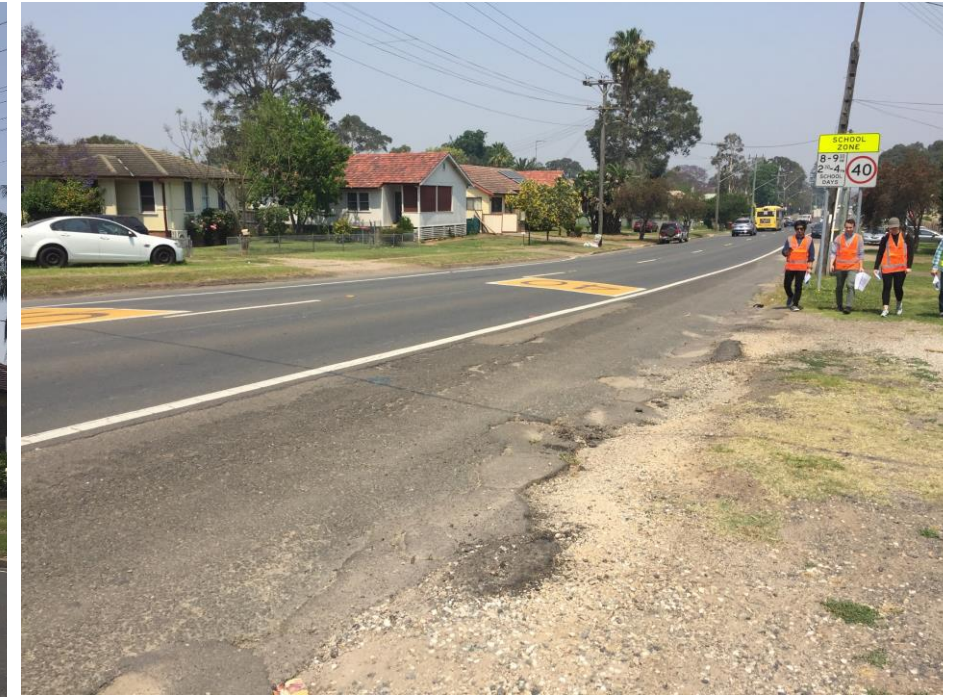
Photo 9 looking southwest down Garfield Road East, note difference between asphalt in road verge and road surface.
