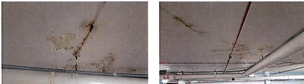
Figure K2: More previously installed failed injection repairs with leaching forming
