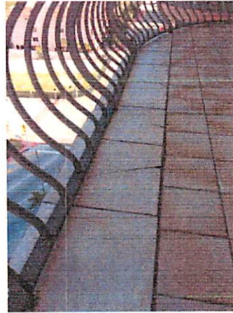
Figure B: Damaged balcony tile that must be removed to fix structural damage
