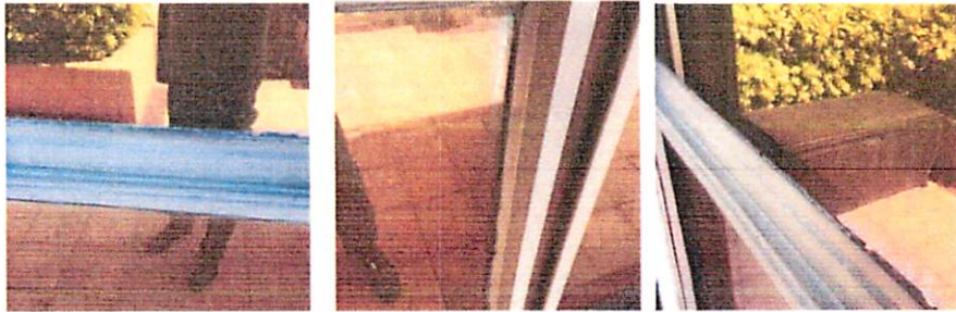
Figure F: Exterior sealant at window frame that has aged past its serviceable lifespan
