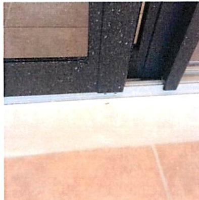
Figure A2: Newly installed sliding door at unit 209 that was not properly flashed
