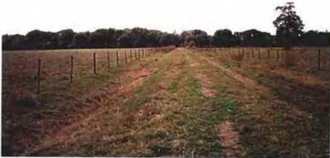
View south of the north portion of East Road where it crosses the northeast pasture. The Banana Creek Canal with trees on the adjacent spoil material is in the background. The road will be elevated and culverts installed to restore west-east surface water sheet flow and adjacent marsh habitat.
