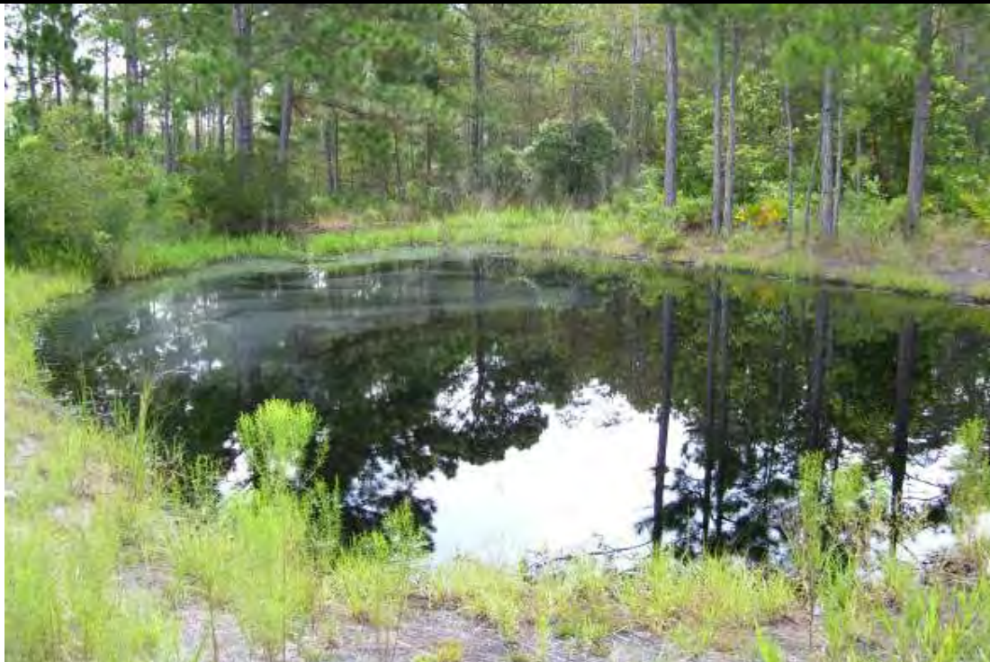
Post-Construction - Site 8 (July, 2009) – the ditch is several hundred feet long, with three small ponds dredged in the ditch footprint to provide fill material necessary to construct two large ditch blocks between each of the ponds. The ponds provide a water source for wildlife during the dry season and the adjacent ditch blocks have stopped the draining of the wetland.
