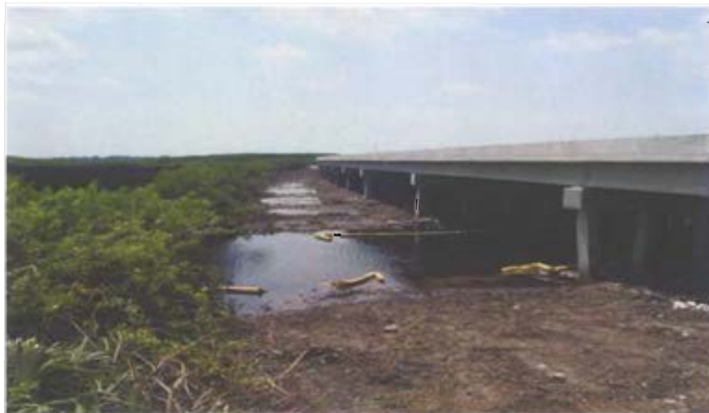
Site A – Post-Construction (Sept. 2003) – the new northbound bridge has been constructed and old bridge removed, exposing bare soil that was under the bridge. The exposed area was planted with white mangrove and black rush.
