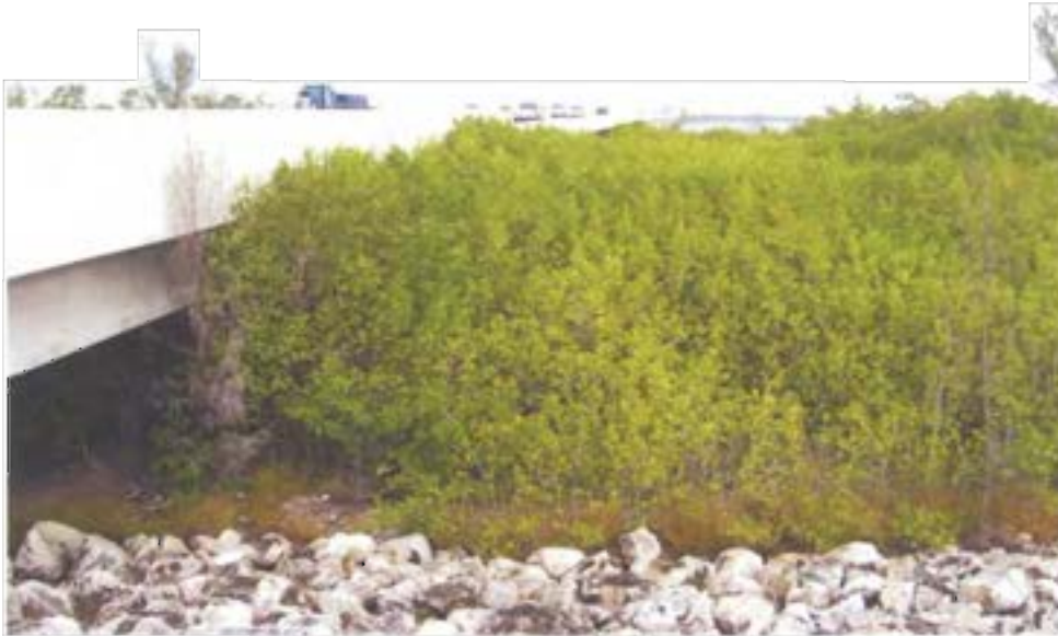
Site C (February, 2008) – following herbicide maintenance in 2004-2005 to help establish vegetative coverage, planted and naturally recruited mangroves have achieved density and heights meeting and in most cases, exceeding pre-construction conditions.
