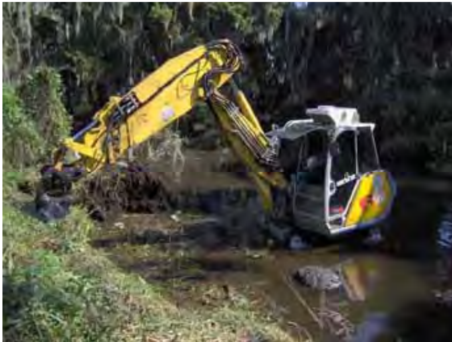
A Menzi unit was utilized in areas where traditional equipment could not access through water, such as this breaching of the rim spoil material to provide hydraulic connectivity to the preserved portion of the Banana Creek Canal.
