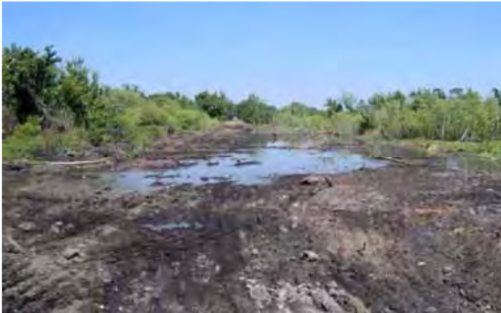
View from the southwest property boundary looking north at the footprint of where the levee was just pushed back into the ditch to restore sheet flow hydrology. The graded area was then planted with hydrophytic plants and trees.
