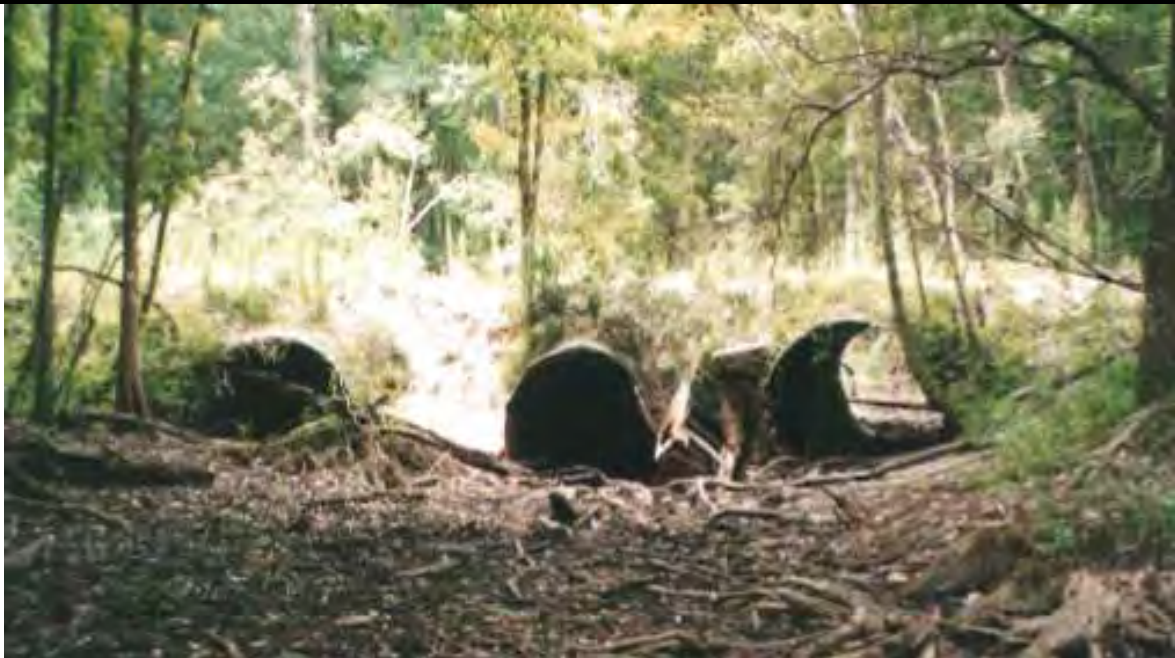
Pre-Construction - Site 2 (2005) – these three dilapidated culverts provide the only hydrologic connections from upstream to downstream through the 700 ft. wide Pithlachascotee River wetland floodplain. The sidebanks of the access road berm are unstable from erosion.
