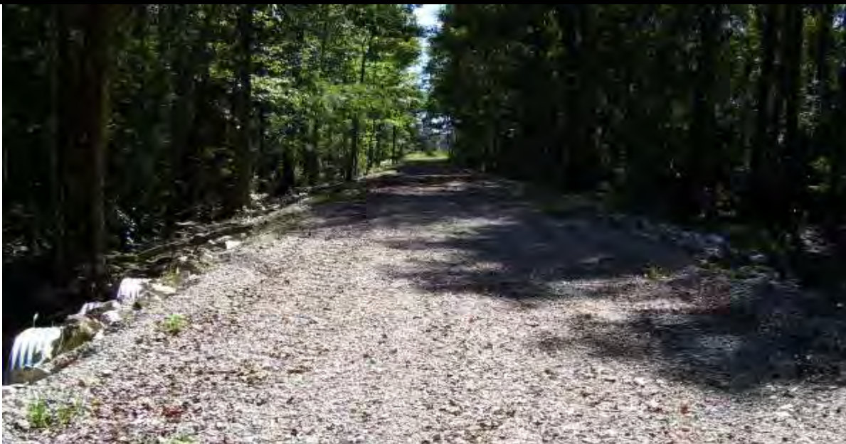
Post-Construction - Site 2 (2009) – in addition to the three new culverts installed at the river channel crossing (left), additional culverts were placed at other strategic locations in the berm to restore appropriate hydrologic regimes and connectivity within impounded wetlands upstream and dewatered wetlands downstream. The access road was stabilized with the installation of rock rubble along the sideslopes and limerock base material on the surface. Wildlife routinely utilize the road for access across the floodplain.
