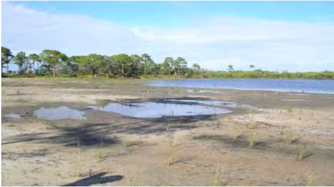
South Tract (2004) – constructed lagoon and planted salt-marsh located within the southeast upland area previously dominated by B. pepper & Melaleuca . Remnant pine flatwood adjacent to Interstate-275 (background) was protected from construction and the habitat enhanced by eradicating exotic vegetation.
