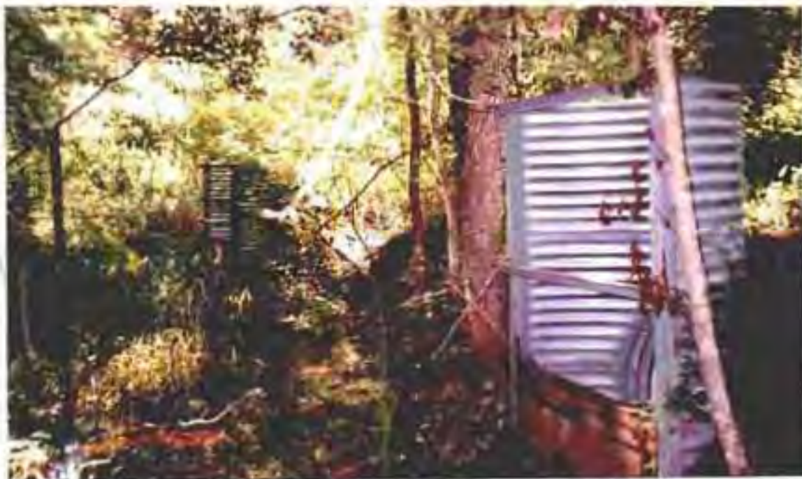
Photo 4 - The two outfall structures with flashboard risers that control the water elevation and flow from Ledwith Lake north to Levy Lake.
