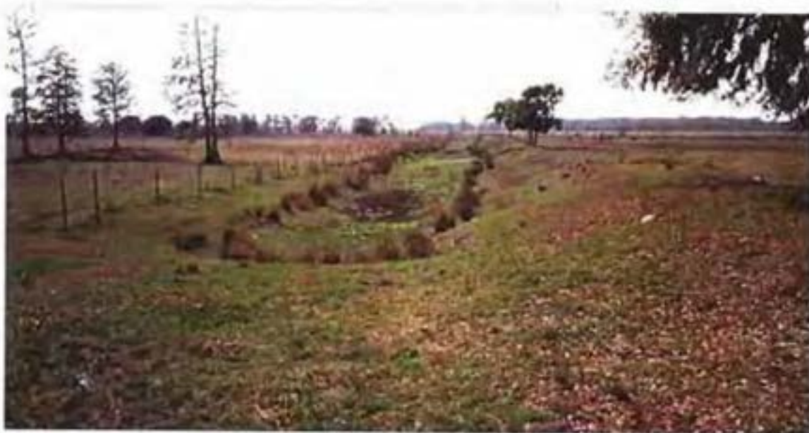
View south from the north end of the remnant and unstable Center Road and adjacent ditch that diverts and drains water south to the Banana Creek Canal. The ditch will be backfilled and clean fill used to reconstruct and elevate the road to restore west-east sheet flow hydrology and adjacent marsh habitat.
