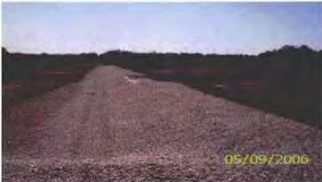
An 810-ft. long discharge weir was constructed to detain surface water, thus restoring the natural hydroperiod of a large slough wetland.
