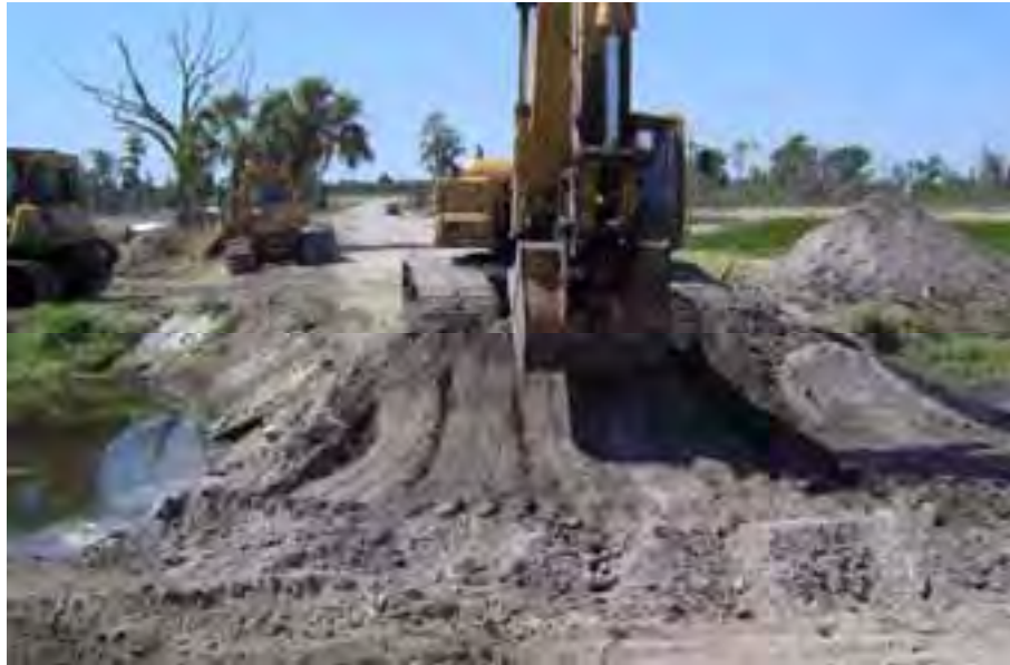
Ditch block construction was conducted where the East Road berm crosses the Banana Creek Canal. This portion of the canal was not backfilled to preserve the existing large oaks and maples along the rim spoil material. The rim material has a hiking trail under the canopy used by both the public and wildlife to gain access around the site.
