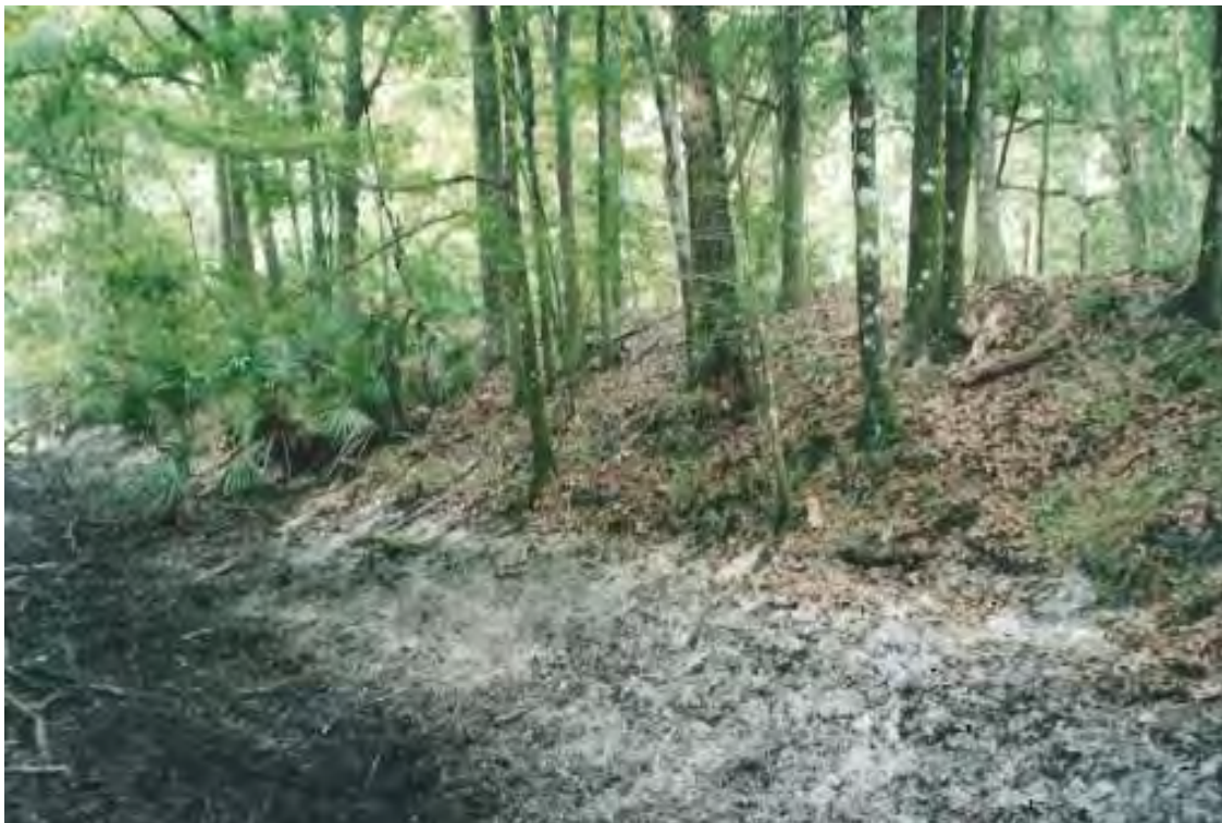
Pre-Construction - Site 4 (2005) – side view of the berm crossing the floodplain. Fill material will be graded back into the dredged donor area (left), elevating and restoring the historic wetland floodplain grade.
