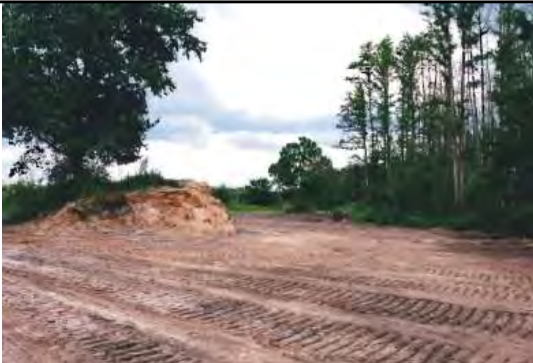
Summer, 2001 – same view of ditch segment after backfilling spoil material into the ditch. Some oak trees (left) were preserved from the earthwork activity.
