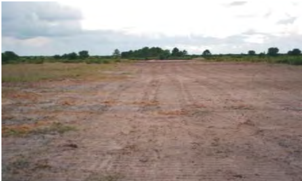
Wetland 6 (Spring, 2002) – same western view over the earthwork area of the graded spoil material and backfilled ditch.
