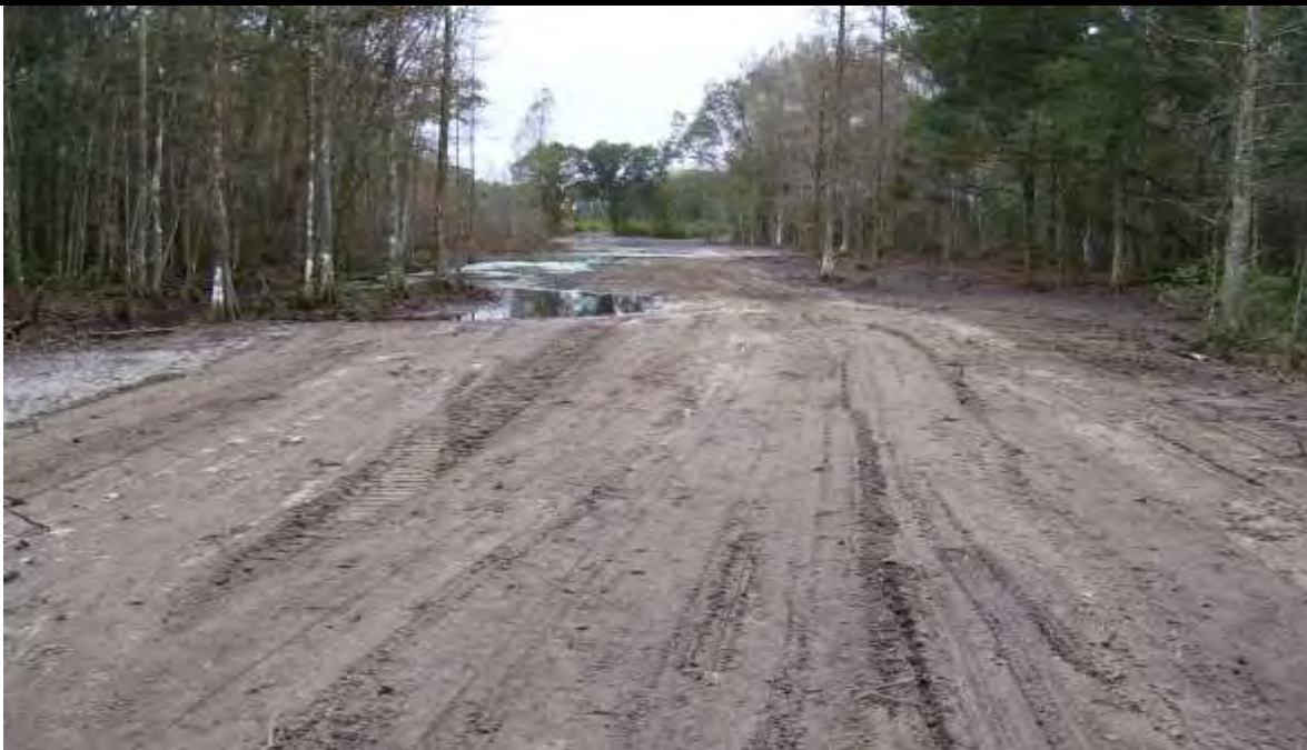
During Construction - Site 4 (February, 2008) – berm material has been graded to fill adjacent ditches, followed by seeding with winter rye and bahia for initial soil stabilization. The base flow through the river channel was maintained, however water sheet flow & seepage has been restored through the floodplain wetland.
