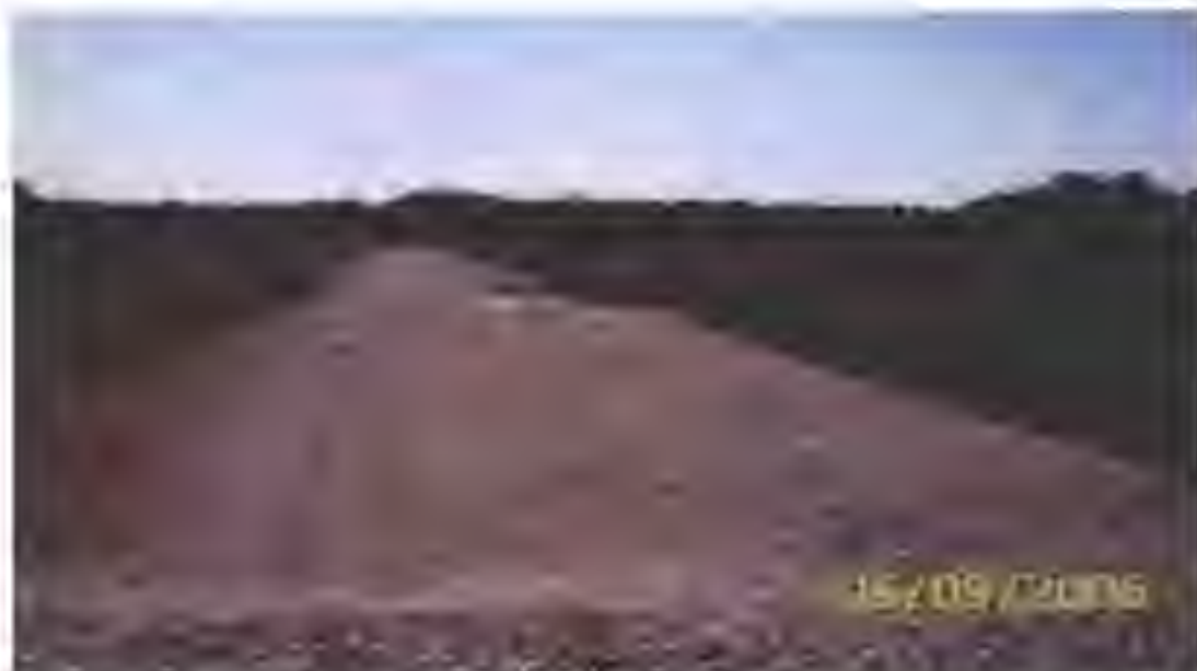
An 810-ft. long discharge weir was constructed to detain surface water, thus restoring the natural hydroperiod of a large slough wetland.
