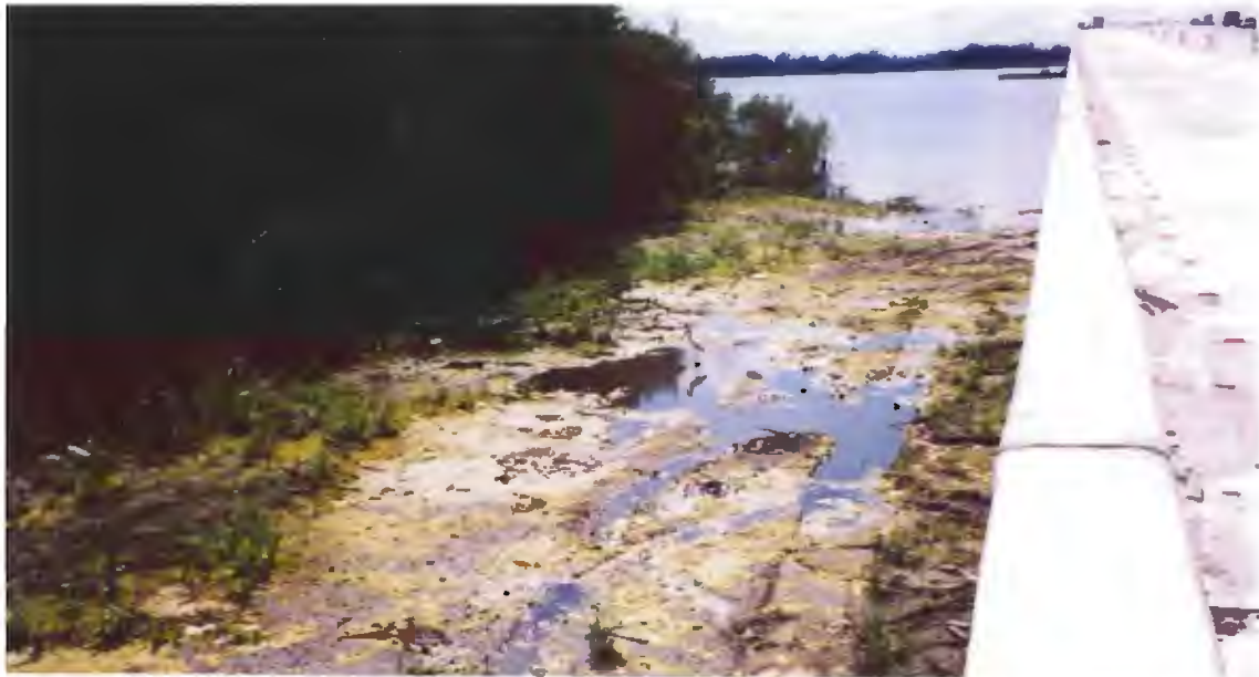
Site B – Post-Construction (Sept. 2003) – the new northbound bridge has been constructed and old bridge removed, exposing bare soil that was under the bridge. None of the large mangroves were impacted, the exposed soil area was planted with white mangrove, black rush and saltmarsh bulrush.
