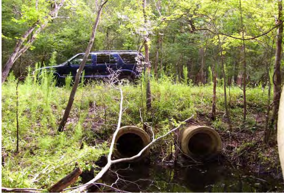
Downstream end of two culverts that discharge water into a creek channel. The culverts will be removed and replaced with rip-rap rubble that will allow gradual seepage into the channel; extending the hydroperiod and attenuation of surface water in the wetland portion on the upstream side of the berm.
