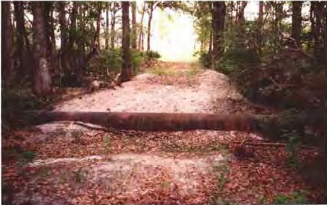
Site 3 – The undersized pipe crossing of Five Mile Creek has resulted in erosion of the fill cap and downstream sedimentation. Further evaluation of this crossing and associated access management will determine whether additional culverts will be installed, or construction of a stabilized wet crossing.
