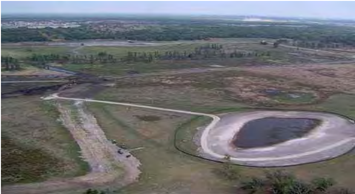
View of the finished Gator Pond, backfilled ditch (left), and Western Access Road during the late stages of construction. Construction equipment moving east to backfill the Banana Creek Canal (center).
