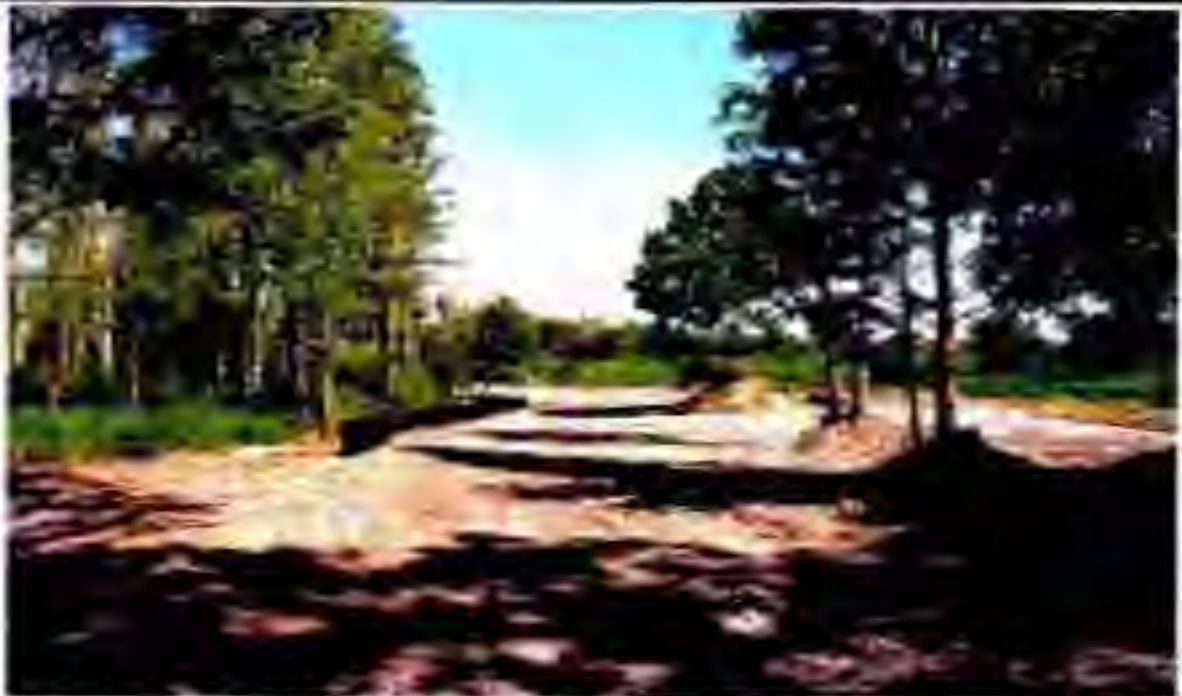
Same view as above photo after spoil material was backfilled. Silt screens installed to minimize erosion into the adjacent wetland while ground cover is establishing. Note where practical, construction worked around the drip line to preserve trees located on previous spoil ridge.
