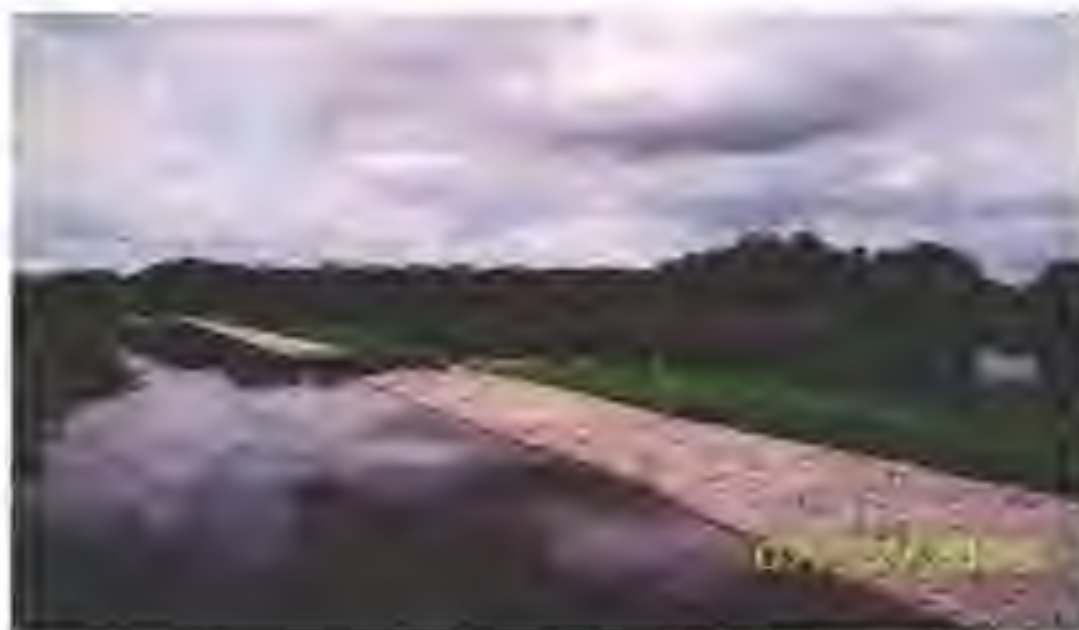
The discharge weir has a combination of two lower discharge elevations constructed with concrete, as seen above at the water overflow in the center of the weir. The broad "overflow" portion of the weir has limerock anchored within 6-inch geoweb containment system. A geotextile liner was placed under the rock to provide additional stability.
