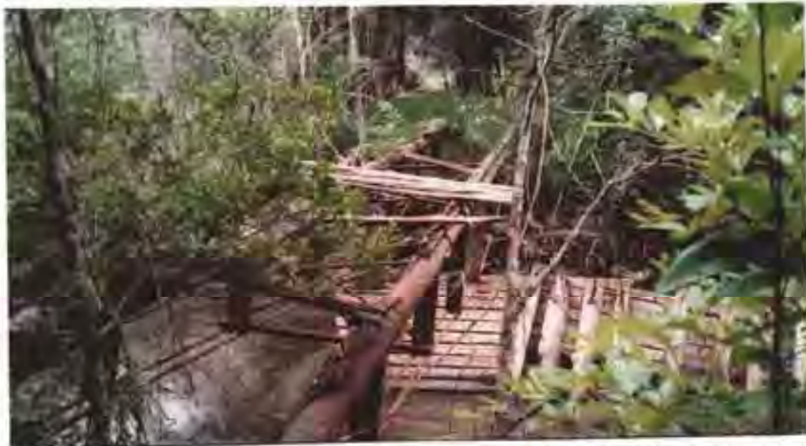
Site 4 – The old tram bridge will continue to decay and eventually fall into the river, which will catch debris, so it will be removed.
