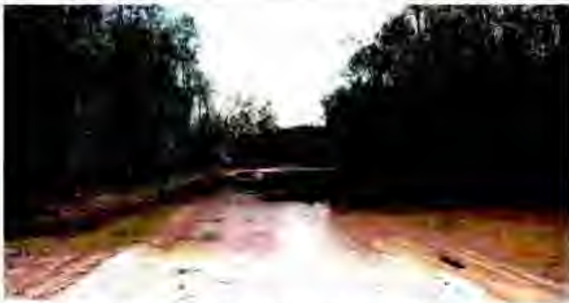
View of the filled east-west ditch and removed tram road, just after construction and prior to tree planting, wetland groundwater and surface water sheet flow hydrology is restored.
