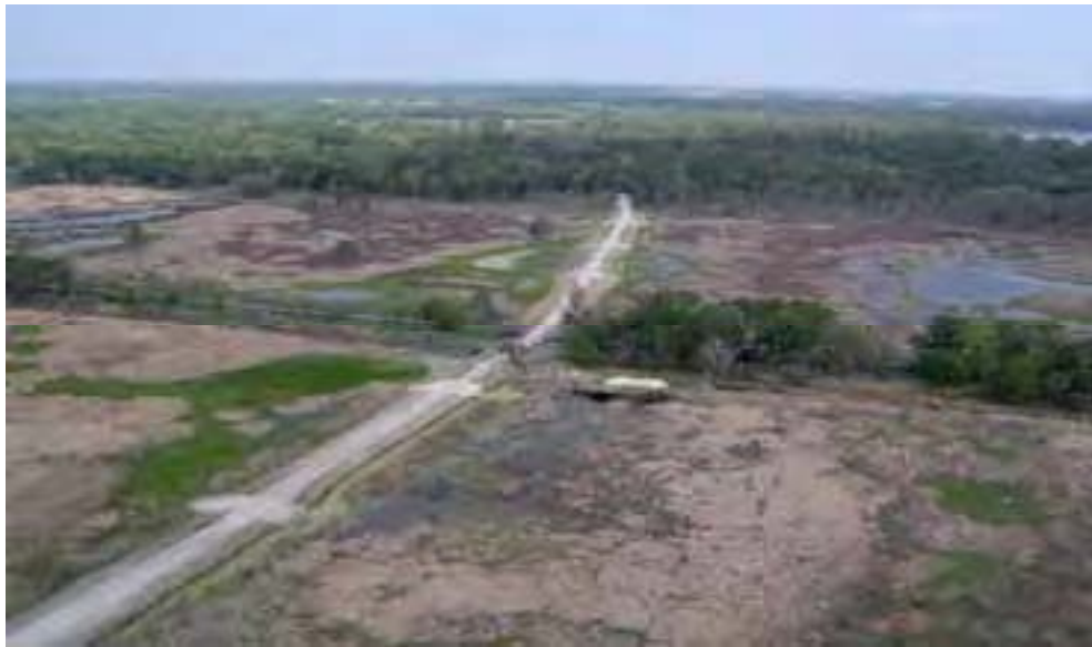
The 2,000 ft. long East Road just after construction. As with the Center Road, the restored sheet flow is evenly distributed by a series of culverts, as well as "saddle" swales installed at lower road elevations to allow overflow during periodic flood events.
