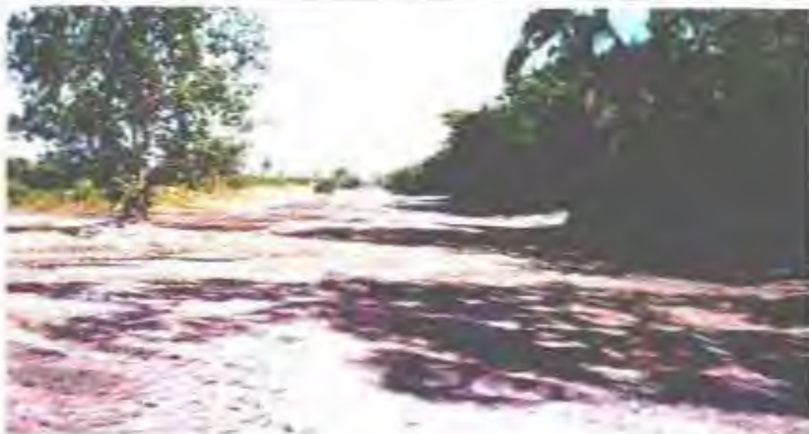
June, 2002 - Wetland 12 – View from the south, looking north at former ditch area (20 feet against tree line) & previous spoil material (center 30 –40 ft.) graded to backfill the ditch.
