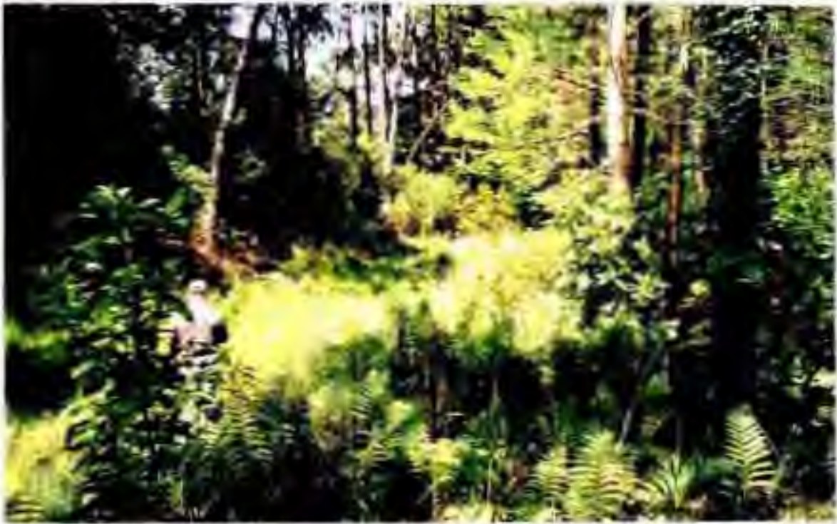
Ditch connecting Wetlands 2 and 4 depict the 5-6 ft. decrease in grade elevation between the Wetland 4 grade (right) and the ditch bottom grade (left).
