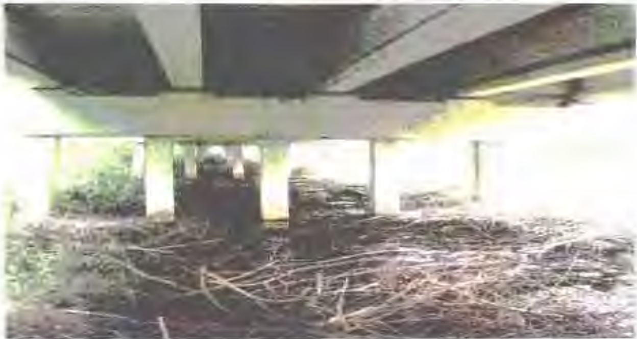
Site C - View under the northbound bridge, minimal vegetation within the area under shade. Once this bridge span is removed, white mangroves are proposed for planting, along with natural generation of mangroves. Stain lines on the bridge pilings indicate normal tidal fluctuations.
