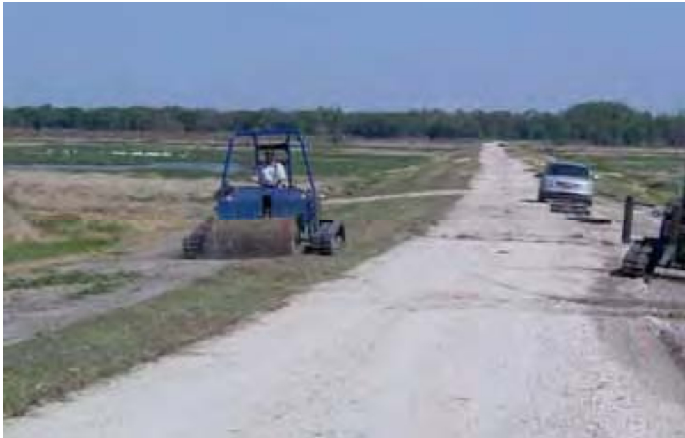
Final construction of the Center Road and sod being installed to stabilize the slopes. Water starting to pool upstream and attracting white pelicans and wading birds (left).
