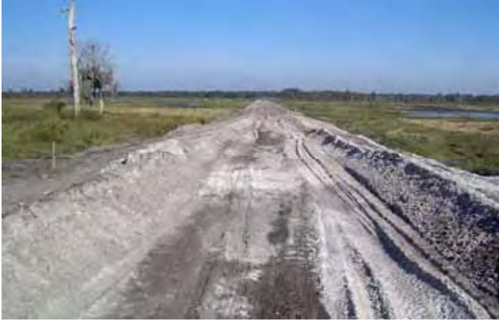
Standing on the southern end of the Center Road looking north. Fill material was used to elevate the remnant road (3,050 ft. long), and culverts installed to restore west-east sheet flow hydrology through the restored and enhanced wetland habitat.
