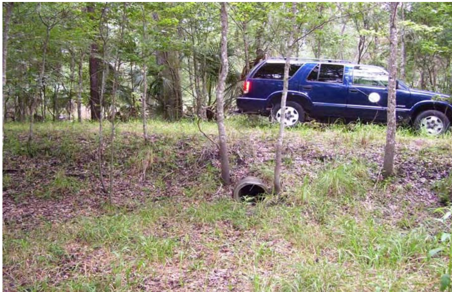
Four of the culverts will remain, however sumps and rip-rap will be placed at the culvert ends to aid in maintaining flow and minimize scouring and undermining of the culverts.
