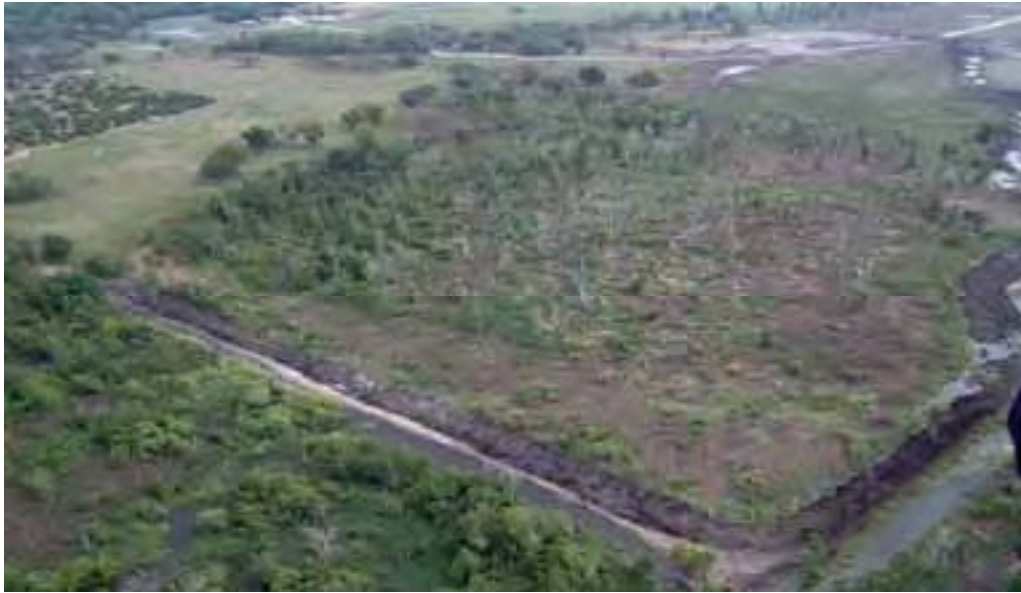
View from the western boundary of the property looking east. The north-south levee (900 ft. long, avg. 5 ft. tall) has just been backfilled into the adjacent ditch to restore western water sheet flow through the remnant forested wetland and proposed forested wetland restoration area. View of a backfilled portion of the Banana Creek Canal is evident along the right side of the photo.
