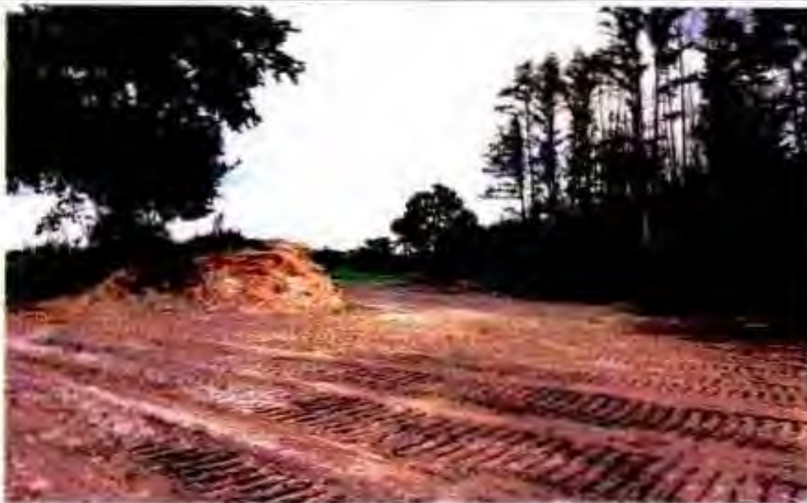
Same view as above photo after spoil material was backfilled. Preserved oak tree (left) on top of spoil mound depicts the amount of graded material required to fill the perimeter ditch.
