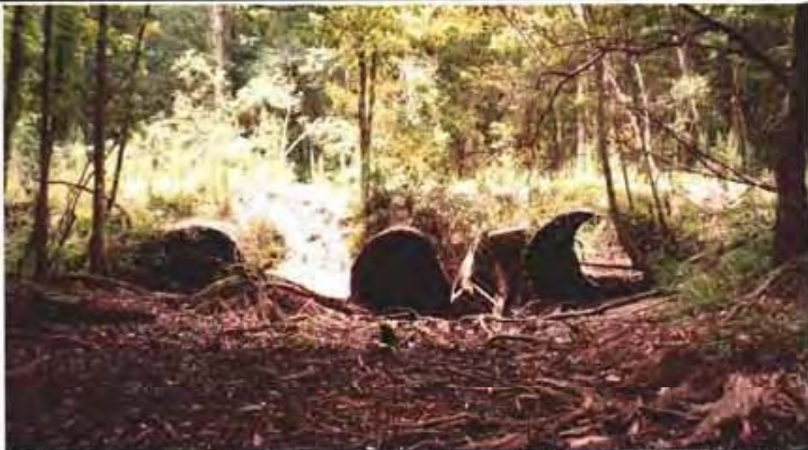
Site 2 – The undersized culverts within the main channel crossing of the Pithlachascotee River. Erosion evident between the center and left culvert, Abandoned refrigerator used as slope stabilization between center and right culvert. These culverts will be replaced with probably more and larger concrete culverts, as well as proper sideslope and pipe stabilization.
