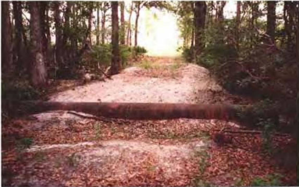
Site 3 – The undersized pipe crossing of Five Mile Creek has resulted in erosion of the fill cap and downstream sedimentation. Further evaluation of this crossing and associated access management will determine whether additional culverts will be installed, or construction of a stabilized wet crossing.
