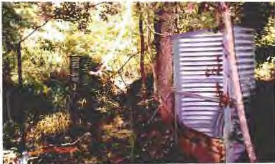
Photo 4 - The two outfall structures with flashboard risers that control the water elevation and flow from Ledwith Lake north to Levy Lake.
