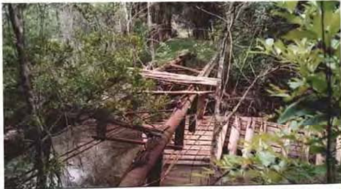
Site 4 – The old tram bridge will continue to decay and eventually fall into the river, which will catch debris, so it will be removed.
