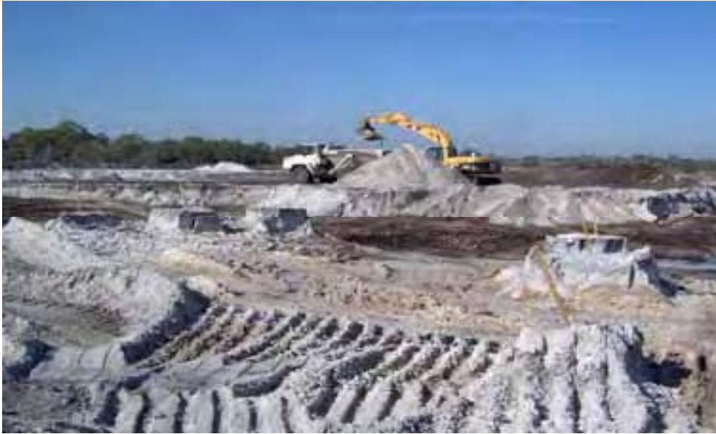
View of the southwest Gator Pond during earthwork activities. Dredging material used to stabilize the Center and Eastern Access Road berms.
