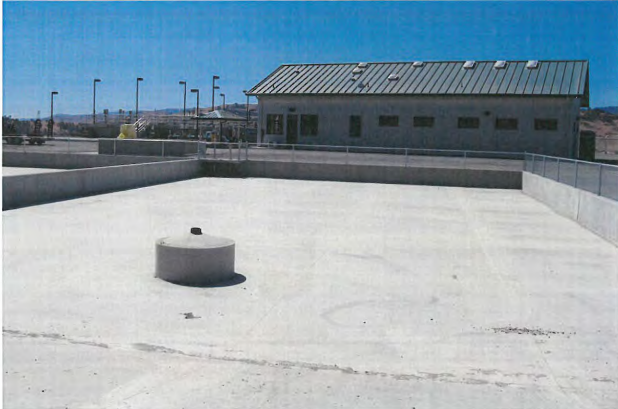
Figure 9-1: Solids Drying Bed #1 (Empty)
