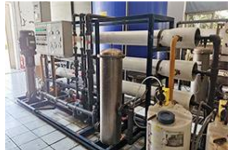
Reuse of wastewater treated by a reverse osmosis membrane system (TRJ)
