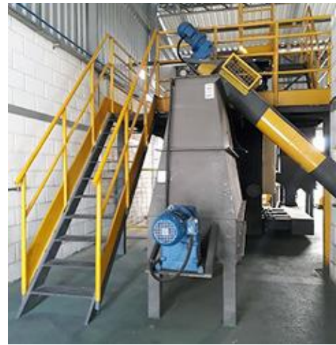
External appearance of a wood-fired boiler (SRK-BI)
