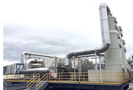
Equipment for treatment of gases generated by vulcanization (TRG)
