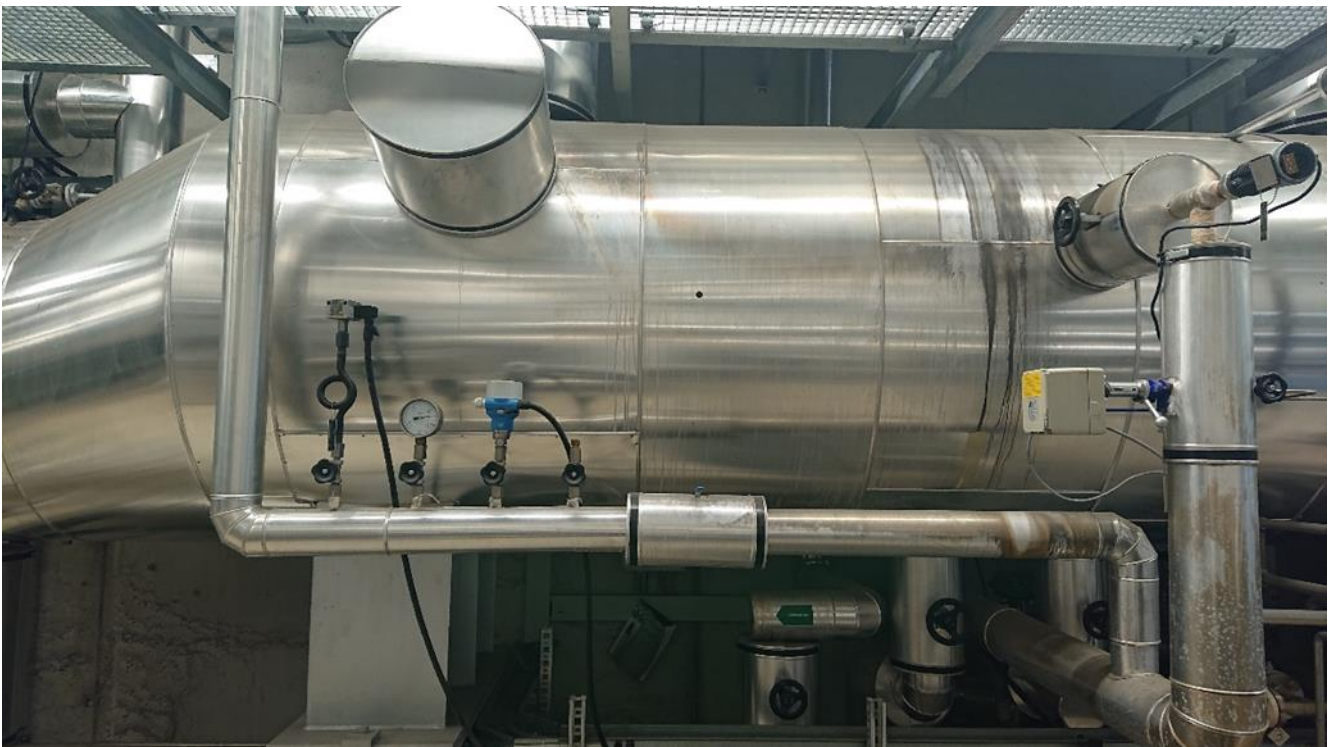
Figure 1: New pressure sensor next to manometerng
