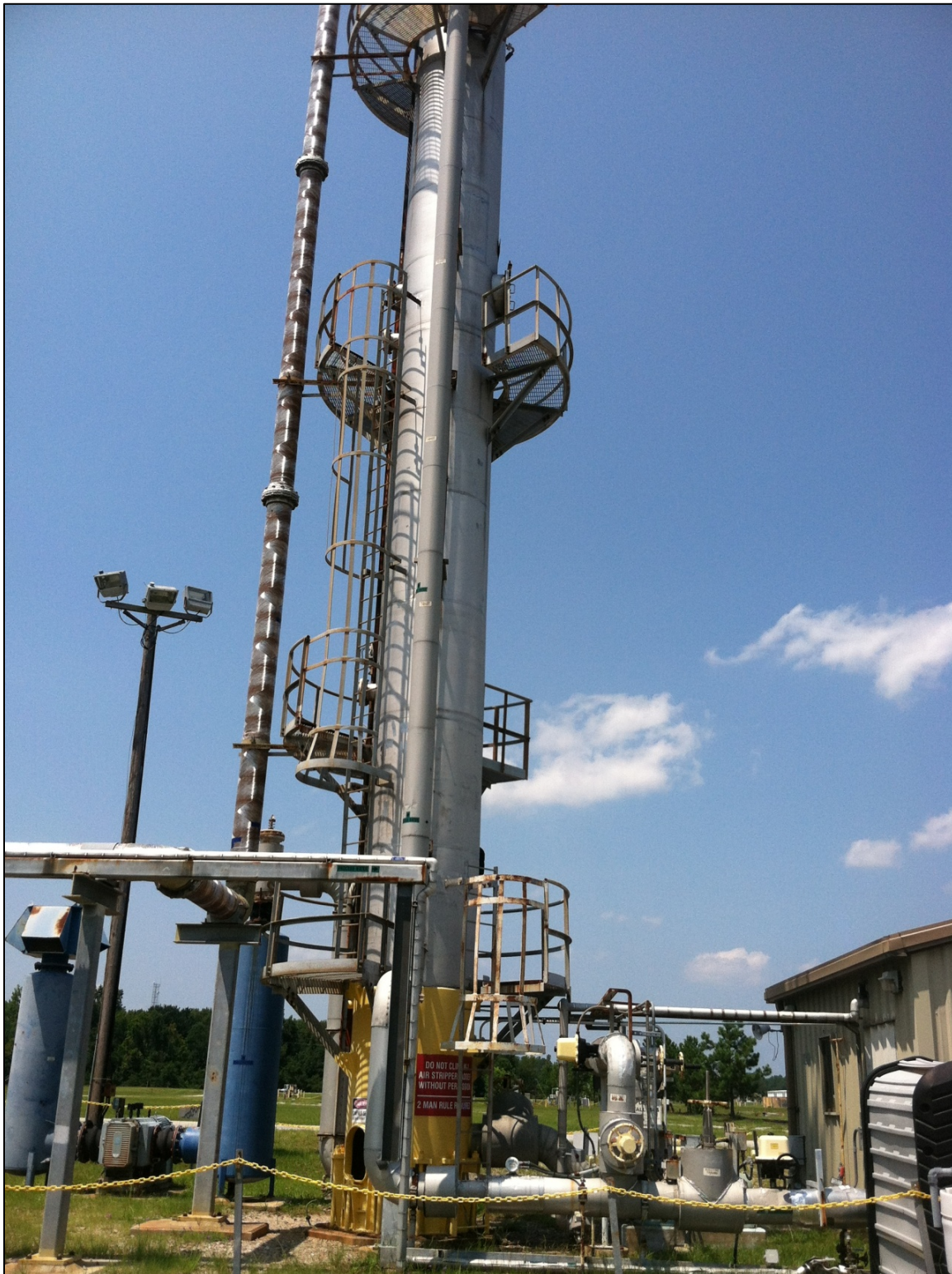
Figure D-4. M-1 Air Stripper System (2017)
