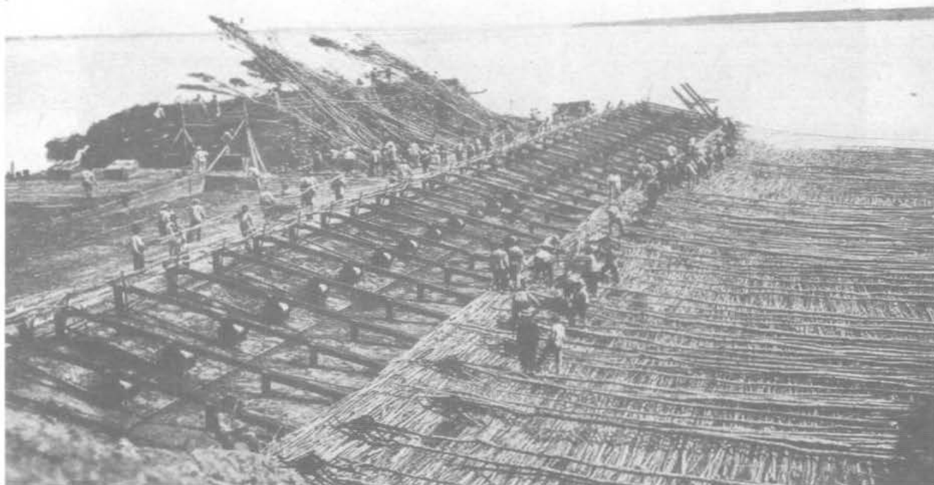
Fig. 6.8. Construction of black willow mats in 1915 for riverbank stabilization in the LMAV. Photo courtesy of J. Stanturf.
