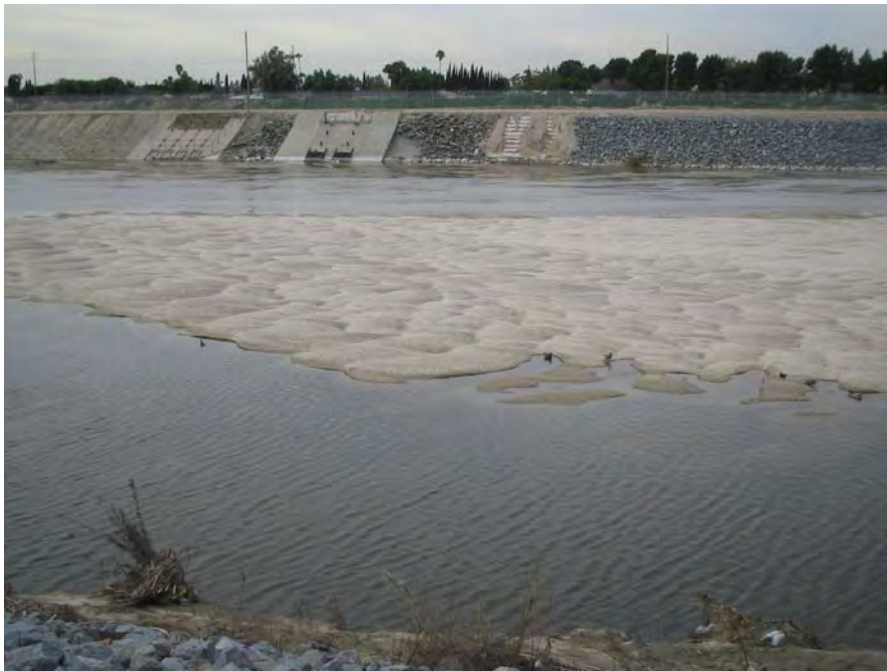
Figure A-5: Sediment Deposition Downstream of Glassell St. and Upstream of the Rubber Dam Structure
