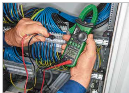
Voltage testing in switchgear cabinet
