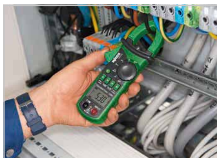
Current measurement in switchgear cabinet
