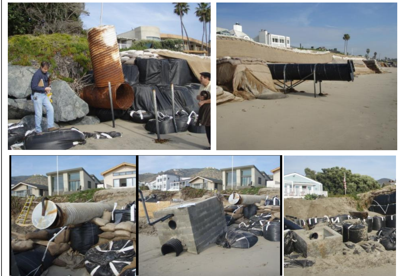
Illustration 3.7-7. Examples of pipes through the revetment. Top row: Storm water drains protruding through sand bag revetment along Broad Beach to drain Broad Beach Road and upland watershed. Bottom row: Construction of a storm drain through the sand bag revetment. Some drains were designed with contained outfalls while others remained as plain pipes draining directly on to the beach.
