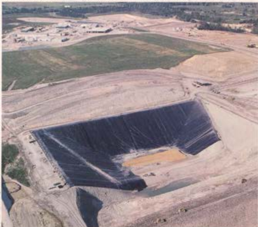
Newly lined trenches will help keep the dangerous poisons in Emelle's wastes from leaking into groundwater—for a short while. The black plastic lining is guaranteed for only a few decades.
