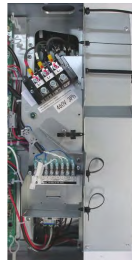
close-up view of terminal block sub-assembly and filter cover
