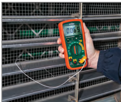
Verify Temperature output on HVAC units using Model EX355
