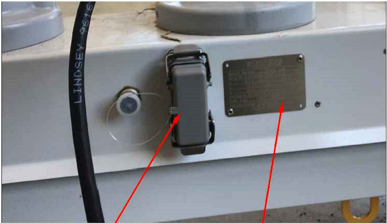
CONTROL CABLE CONNECTOR
