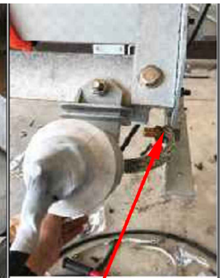
LOAD-SIDE ARRESTOR GROUND
