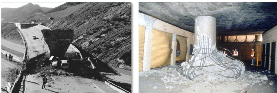
Figure 3.3 – Bridge damage from the 1994 Northridge earthquake event
