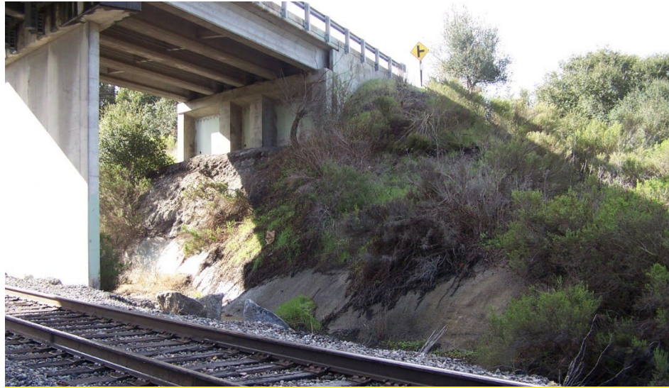
Figure A.5 - Pre-Cast Girders used to span railroads Edna Overcrossing Bridge on Price Canyon Road, San Luis Obispo County, CA
