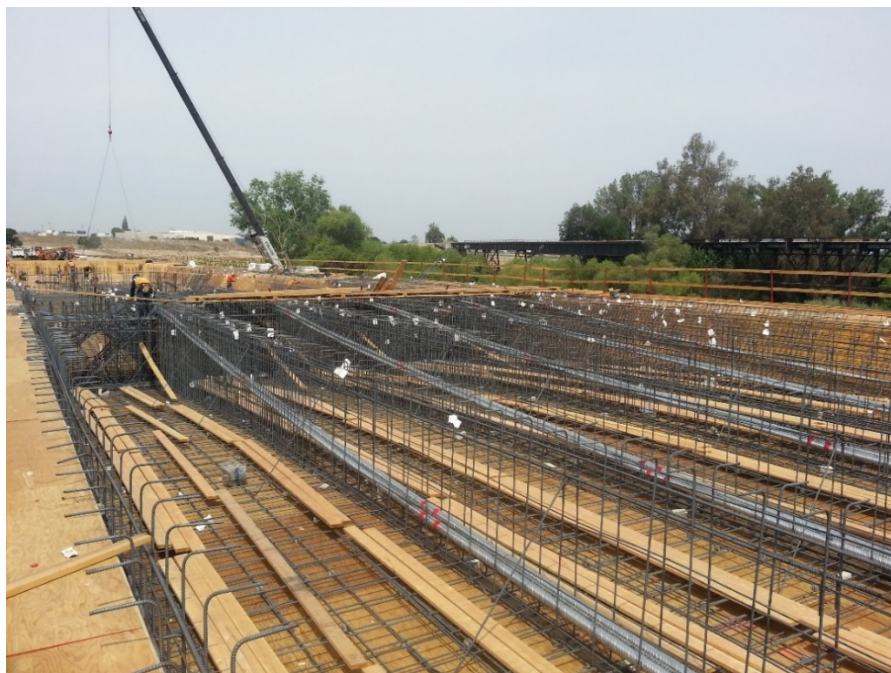
Figure A.2 - Prestressing ducts placed in a cast-in-place box girder bridge Manning Avenue over Kings River Bridge, City of Reedley, CA
