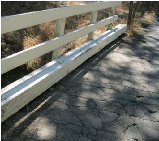
Figure 4.10 - Bridge Deck Requiring Replacement
