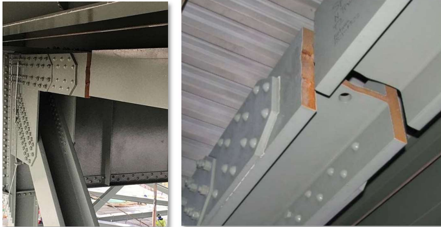
Figure 3.4– Fracture of main steel truss member on the Delaware River Bridge in 2017. Investigation determined the cause was due to welding repair practices at the time of construction in 1956.
