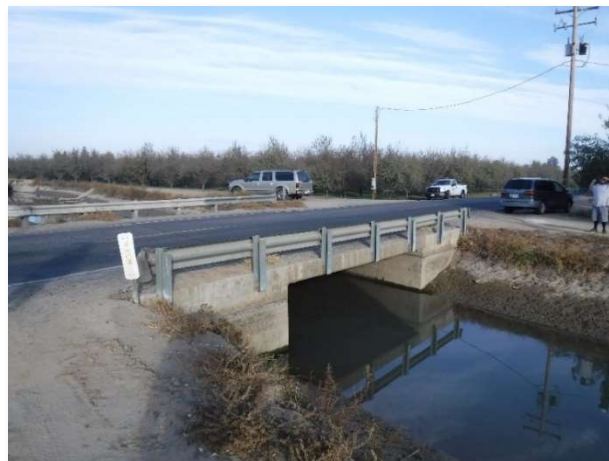
Figure 2.2 – Cressy Way Structure at Livingston Canal in Merced County. This structure does not meet the federal definition of a Bridge, though it performs the same function for it’s respective road network.
