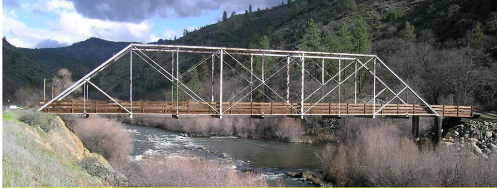
Figure A.7 - Historically Significant Steel Truss Bridge (Replaced) Klamath River Road over Klamath River, Siskiyou County, CA
