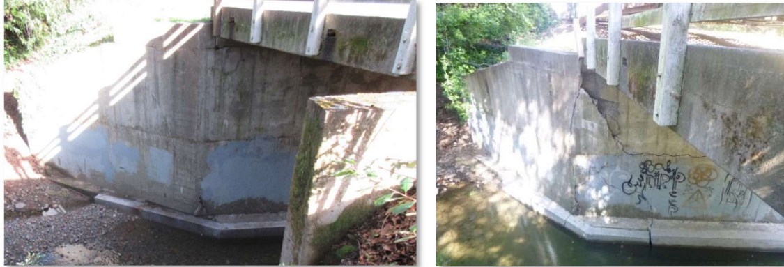
Figure 4.12 - Progression of Bridge Foundation Damage from Scour Over 2-year period at Robinson Creek Bridge in Mendocino County
