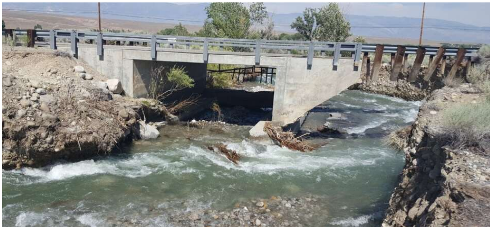
Figure 3.5 – Scour Damage to the Round Valley Bridge in Inyo County in 2017
