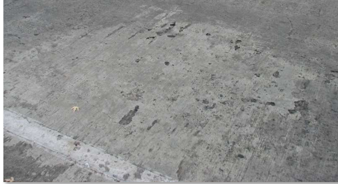
Figure 4.9 - Bridge Deck Requiring Rehabilitation
