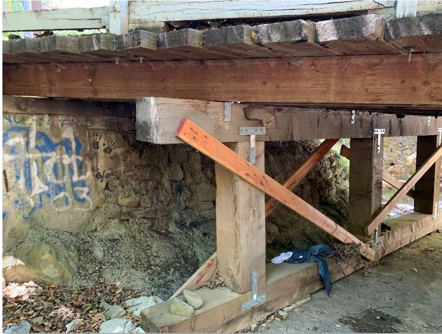
Figure 4.14 - Temporary Timber Support Used to Increase Load Carrying Capacity. This Older Bridge is in Good Condition but Not Able to Carry Modern Vehicular Loads.
