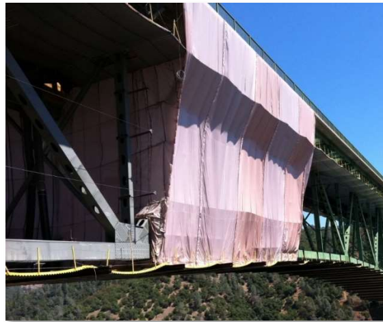
Figure 4.8 - Global Lead Containment System Auburn Foresthill Bridge on Foresthill Road over the American River in Placer County, CA
