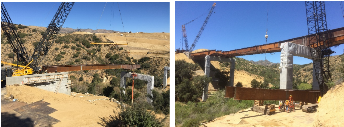
Figure A.6 - Steel plate girder bridge erection Poema Avenue over Devils Canyon Creek, Los Angeles County, CA
