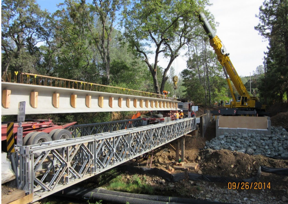
Figure A.3 - Pre-cast Girder Bridge Erection Hilderbrand Drive Bridge over Saint Helena Creek in Lake County, CA
