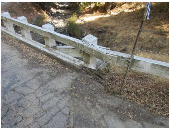
Figure 2.6– Bridge Deck in poor Condition, Morgan Territory Road, Contra Costa County
