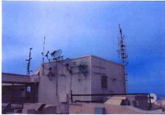
Existing Telecommunications (not Sprint-owned)
