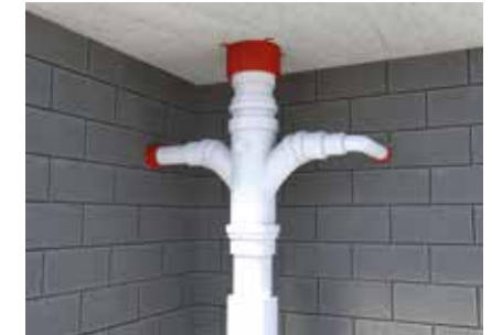
Pipework and Trunking
