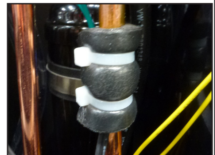
Thermistor attached to the refrigerant line.
