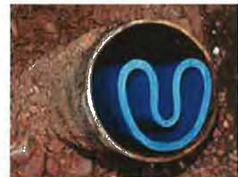
Figure A4-5 Deformed Pipe
